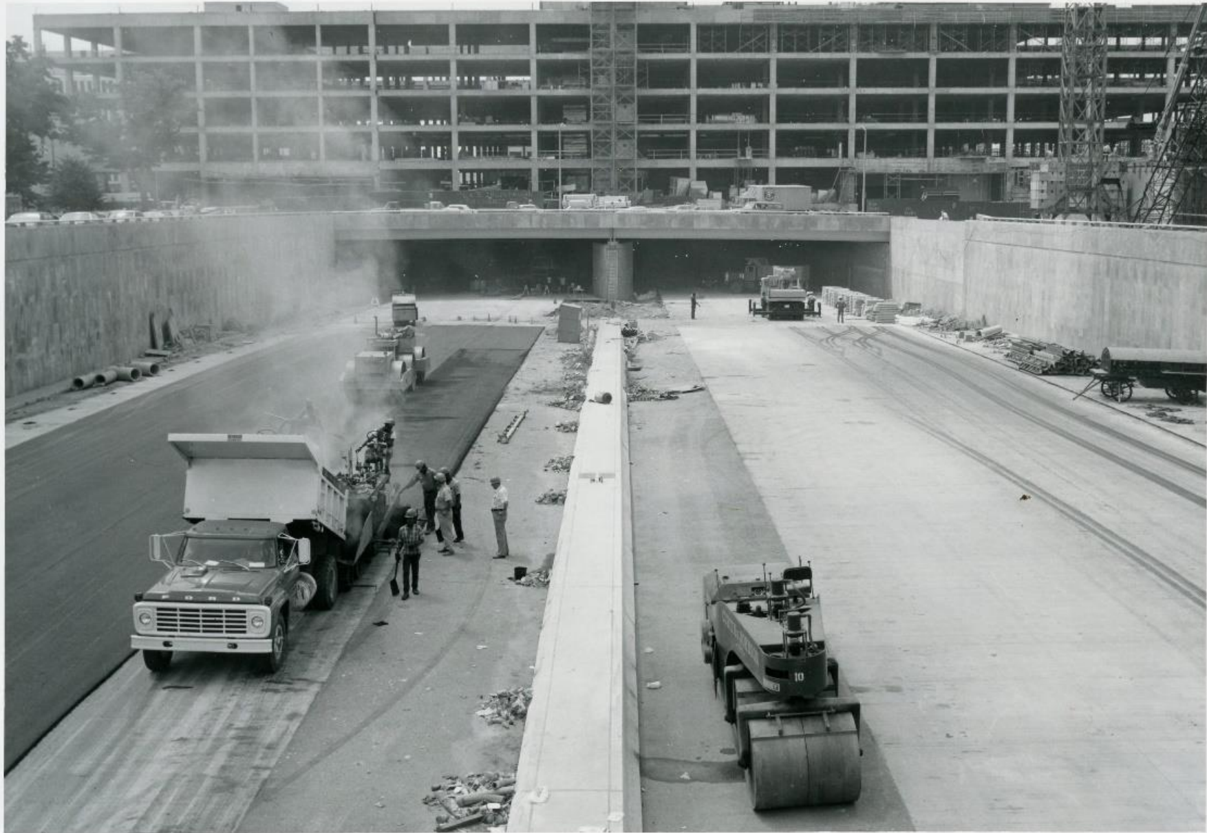
CENTER LEG OF INNER LOOP - D S T. S. W. TO MASS. AVE. N. W. MALL TUNNEL - CONTRACT NO. 6
